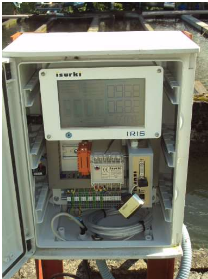
Outdoor (IP66) cabinet tailored telecontrol outstation in a plug & play industrial execution.
